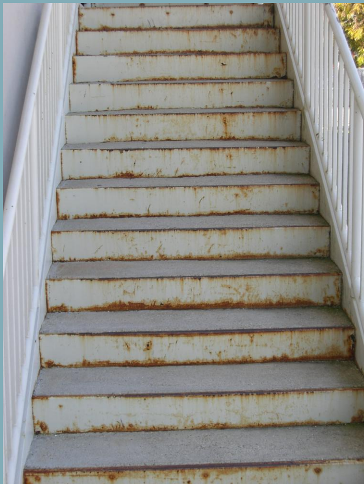
Rusting stairs at UCA's Caldwell Apartments in downtown Conway, AR
