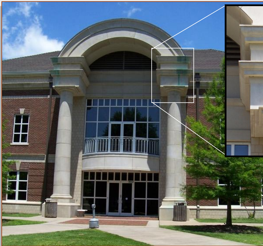
South-facing entrance of Harrin Hall (UCA). Corrosion from copper sheathing over the arched door runs down the face of the column as blue-green streaks.
